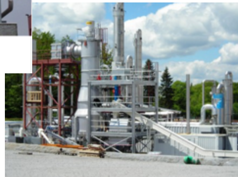
Wood Fuel and/or Distillery Residue Gasification System – 2006 | Europe
