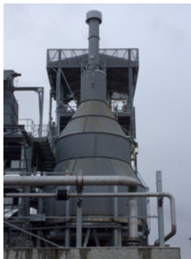
RDF, Wood & Wood Waste Gasification – 2014 | U.S.A.
