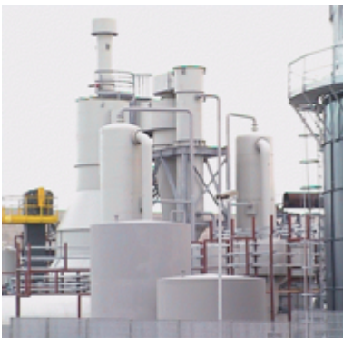
Olive Residue Gasification – 2001 | Europe
